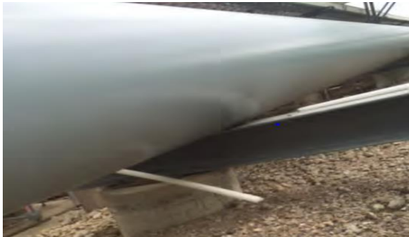
Plastic Rod Failure: Rod Completely Detaches
