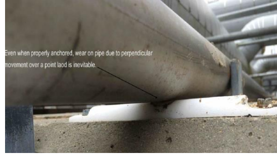
Plastic Rod Failure: Pipe Damage
