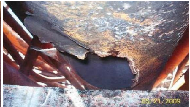
Welded Metallic Saddle Failure
